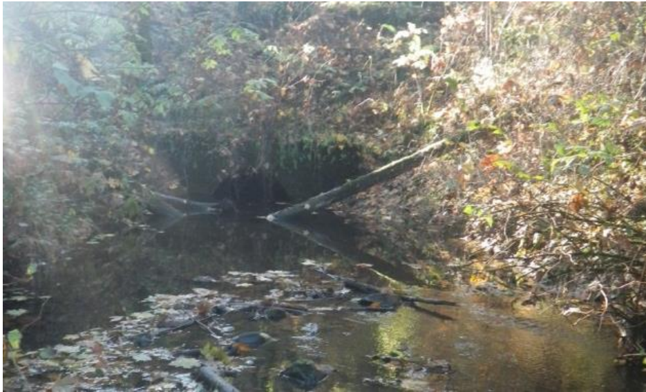
Figure 15. A semicircular culvert located under Highway 30 at the upstream end of reach 1 of McBride Creek, near Columbia City, OR, in December 2012.
