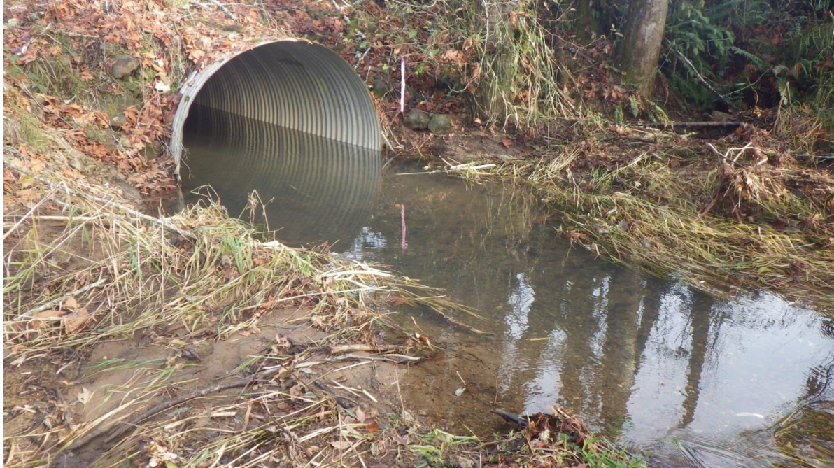
Figure 169. A circular culvert, under a logging road, located at the upstream end of the reach on North Fork Stewart Creek (picture taken in the fall 2012).
