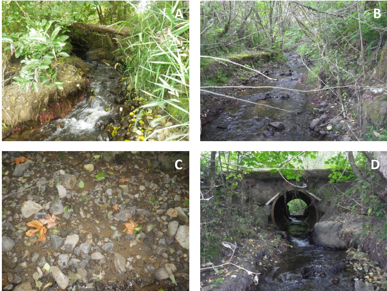
Figure 161. Survey pictures on OK Creek show a riffle (panel A), entrenched channel along the stream banks (panel B), substrate section with > 50% fine sediment (panel D), and a circular culvert under Colvin Road (panel D).
