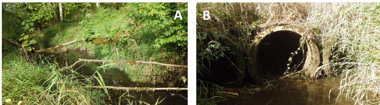
Figure 167. Survey pictures of Stewart Creek show a tidal channel downstream from the reach (panel A) and three adjacent circular culverts under Rutter Road (panel B).
