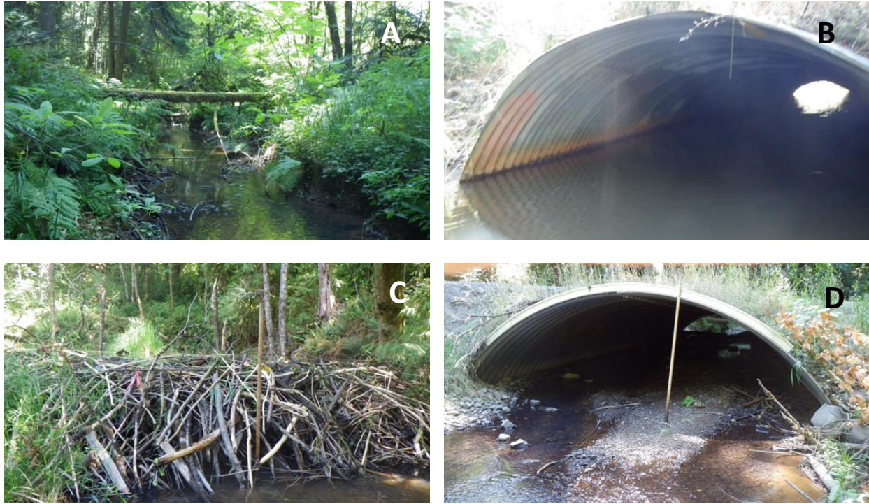
Figure 45. Survey pictures on Salmon Creek showing the dense riparian vegetation in the upstream end of the reach (panel A), a circular culvert at the second Brinn Road bridge (panel B), a large beaver dam (panel C), and a semicircular culvert at the third Brinn Road bridge near the upstream end of the reach (panel D).
