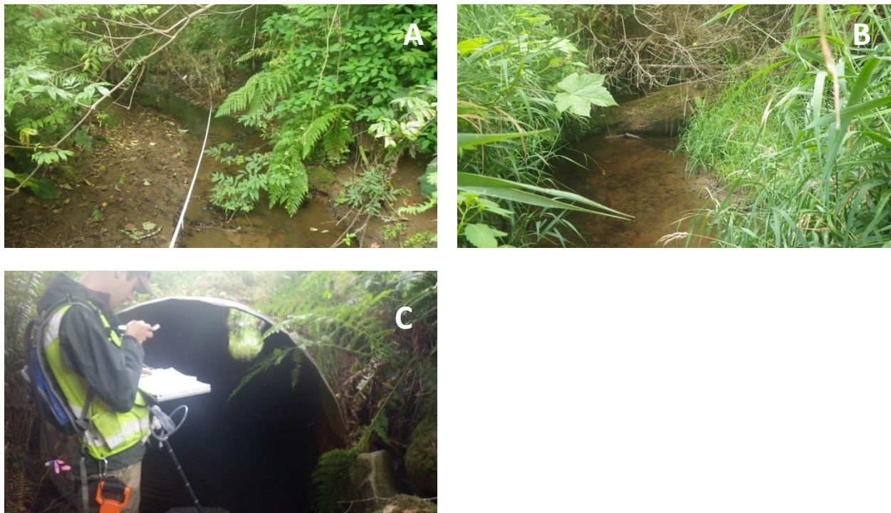
Figure 102. Survey pictures on reach 1 of Hillcrest Creek showing dense riparian vegetation consisting of shrubs, grass, ferns and sparse trees (panel A), the streambed filled with mud and silt (panel B), and a semicircular culvert located near the upstream end of the reach (panel C).
