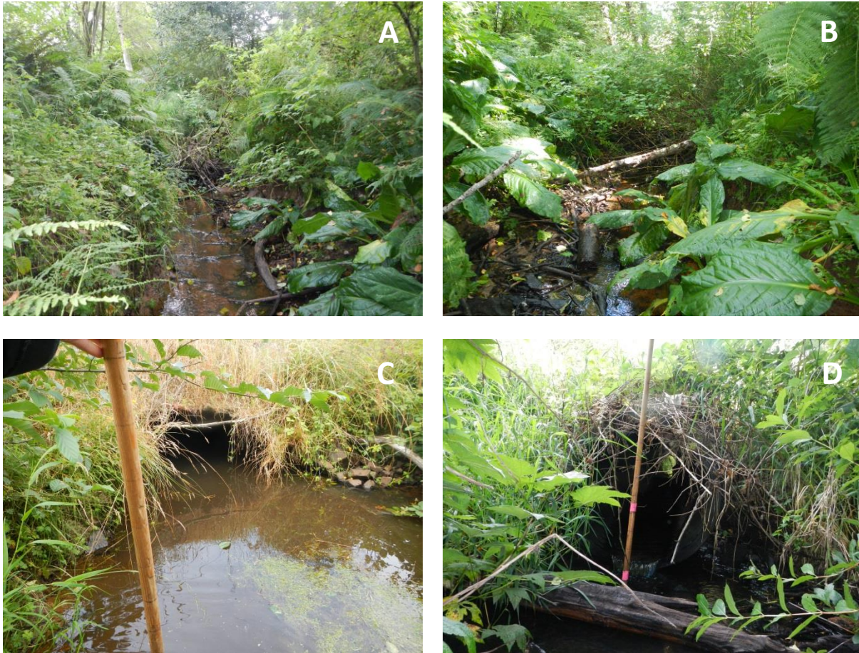
Figure 3. Survey pictures on Barrett Creek show a riparian zone dominated by alder and shrub (panel A), substantial quantities of woody debris within the stream channel (panel B), a semicircular culvert under Lewis and Clark Road located at the downstream end of the reach (panel C), and a circular culvert under Conifer Lane located at the upstream end of the reach (panel D).
