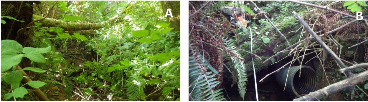
Figure 107. Survey pictures of an unnamed tributary of Hillcrest Creek show a densely-vegetated riparian zone with shrubs, ferns, alders, and maples (panel A) and a crushed circular culvert at the upstream end of the reach (panel B).
