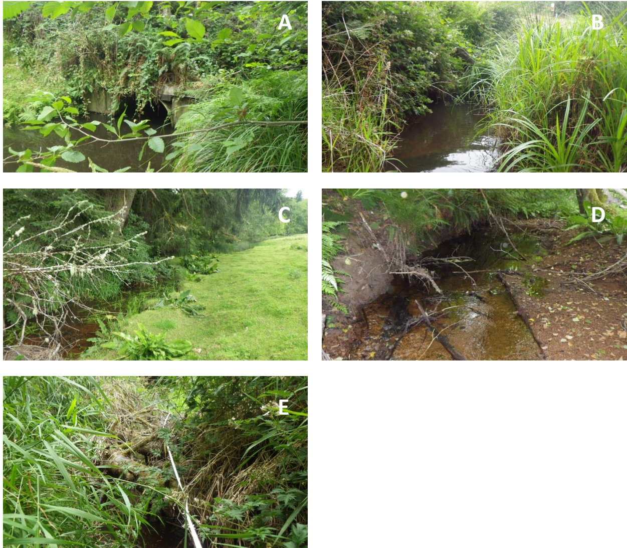
Figure 7. Survey pictures on Johnson Creek showing a circular culvert downstream of the reach start under Loukas Lane (panel A), a slough channel downstream from reach 2 (panel B), dense brush and grass along the stream channel in reach 2 (panel C), a streambed consisting of silt and mud (panel D), and dense woody debris within the stream channel (panel E).
