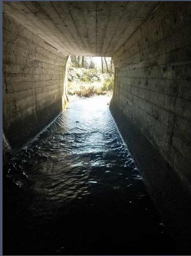
Long undersized culvert
