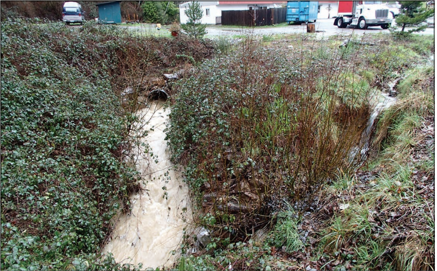
Top photo shows the outlet of the Riverside Market culvert, the segment of open stream channel, and erosion in the county road ditch that results when the stream diverts. The bottom photo shows the Chetco River backwatering the outlet channel below the county road. Note the contrast between the backwater and the segment of open stream channel, with respect to refugia.
