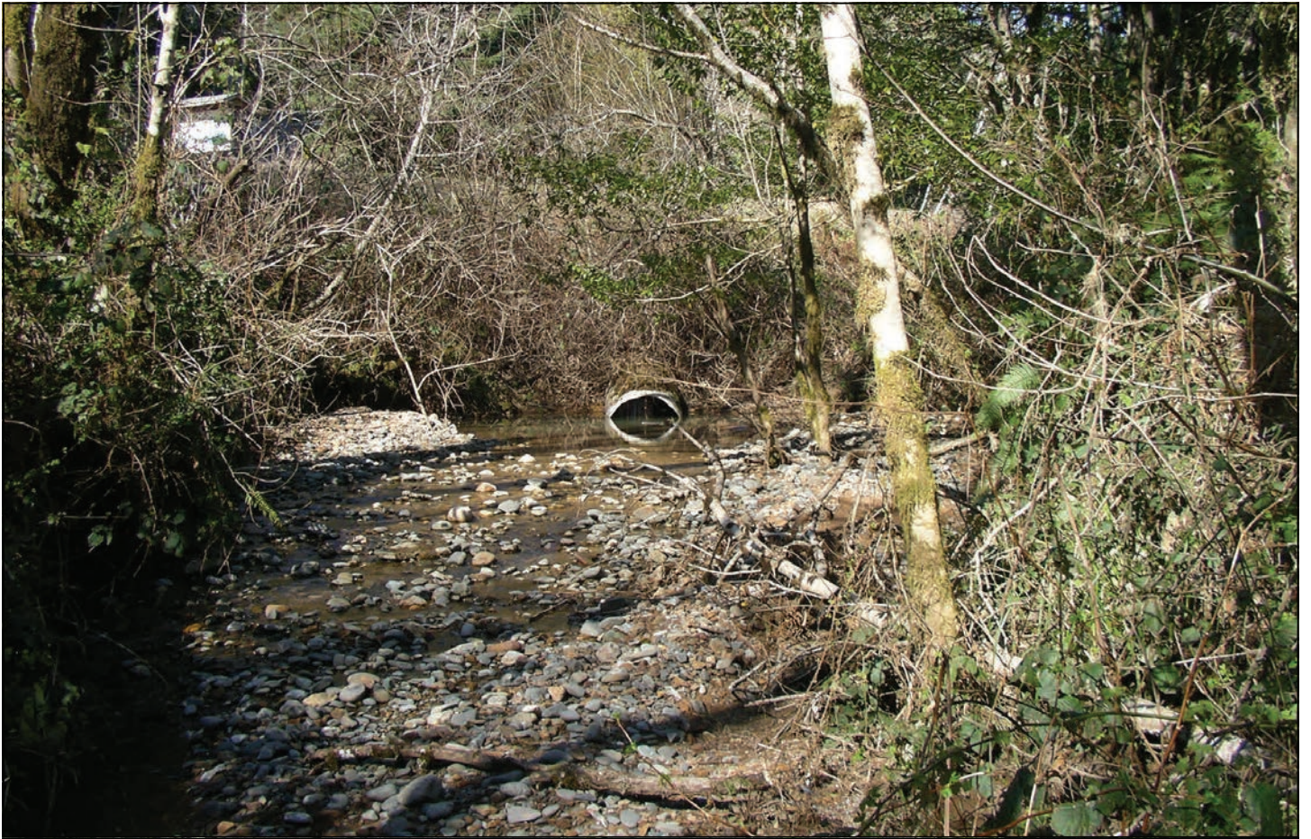
Top photo shows the outlet of the County Road culvert, which is bowed and partially submerged. The bottom photo shows the inlet of the County Road culvert and the segment of open stream channel that exists between the two culverts.
