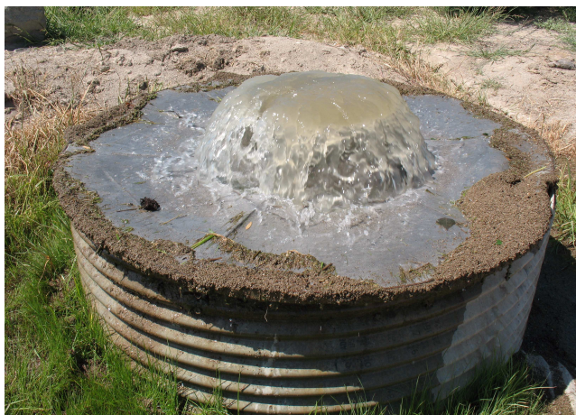
Figure 7.10. Debris in the water is removed by the weed screen and won't clog subsequent parts of the irrigation system.
