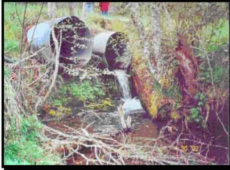
Figure 1 Old culverts on Lee Creek. Note three-foot drop at outlet.
