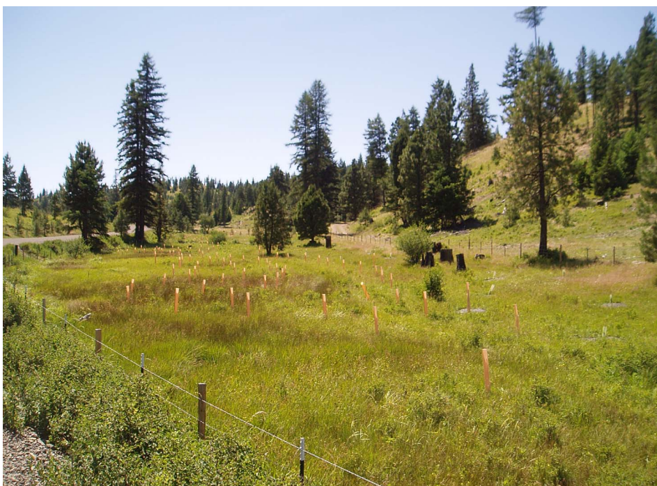
Figure 5.8. Riparian zone restoration occurring in Davidson Canyon in the upper portion of the Rock Creek watershed in Morrow County, Oregon. Tree seedlings have been planted throughout the area in the photograph. Also note the fencing on each site of the riparian area that effectively excludes cattle and has promoted regeneration of lush grasses and other herbaceous vegetation.
